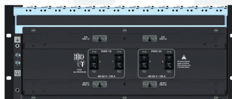
Two feeds non-redundant for 500W/slot
