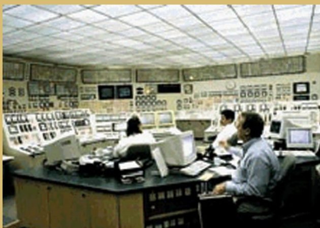
Plant Control Room at Ameren Callaway Facility
