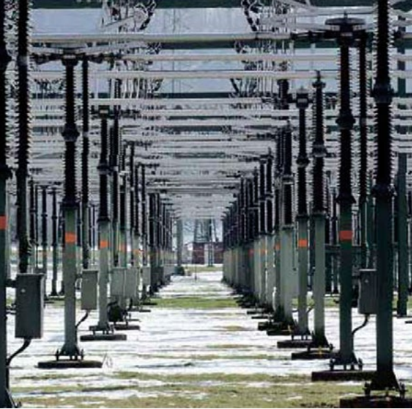
Power Transmission Lines Switzerland
