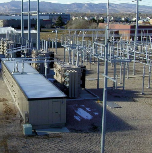
Fort Collins Utilities Monitored Substation
