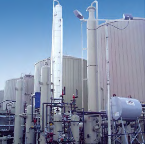
Microgy's Digester Equipment
