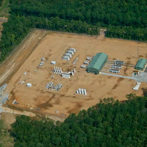
ENSTOR's Caledonia Facility
