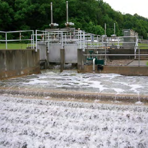
Water Treatment Plant in Operation
