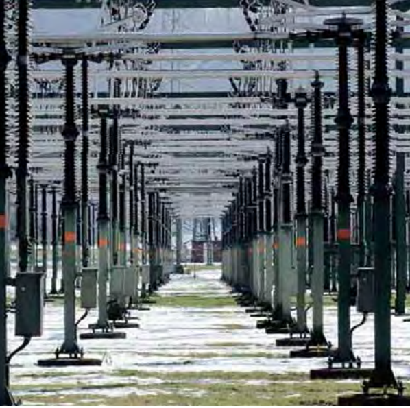
Power Transmission Lines Switzerland
