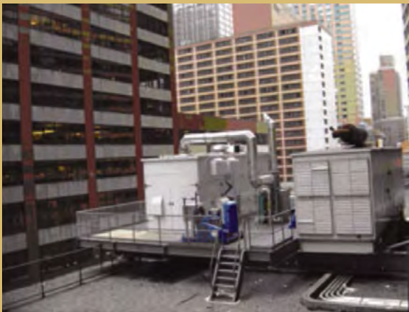
A DFC300 Installation in Downtown Manhattan
