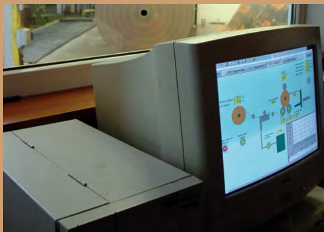
Final Control Process Station
