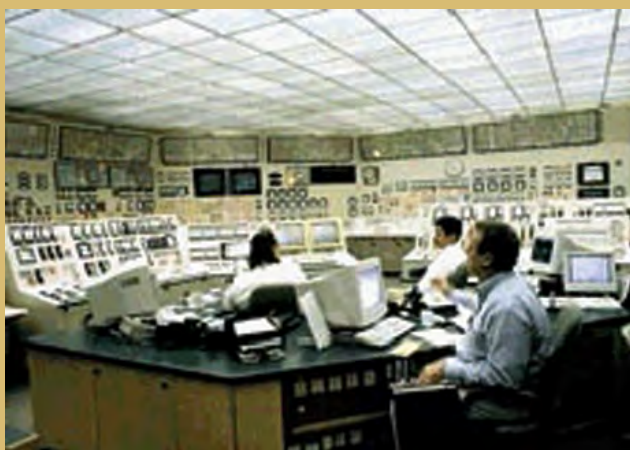
Plant Control Room at Ameren Callaway Facility
