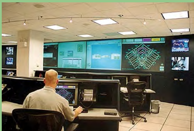
The Pentagon Building Operations Command Center
