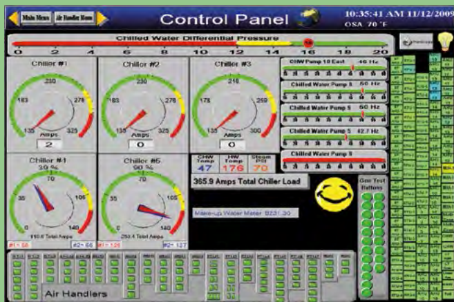
Longmont United's Self-built Control Panel
