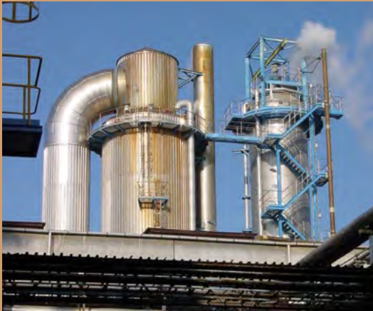
Pulp Processor System at Mondi Packaging
