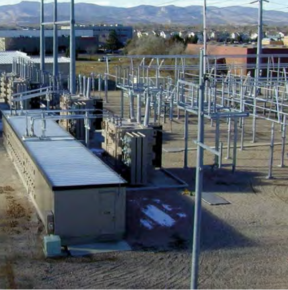
Fort Collins Utilities Monitored Substation
