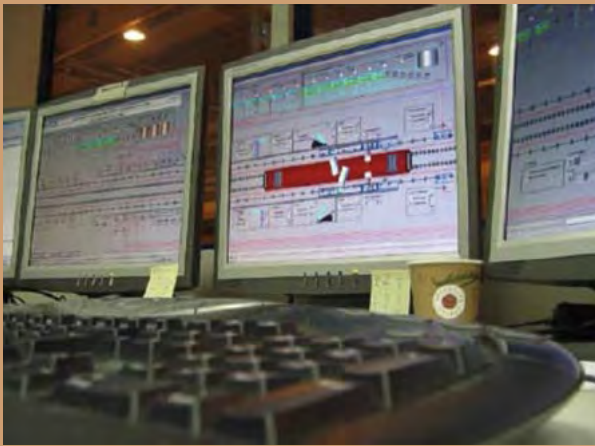
Train Wash Operator Control Area
