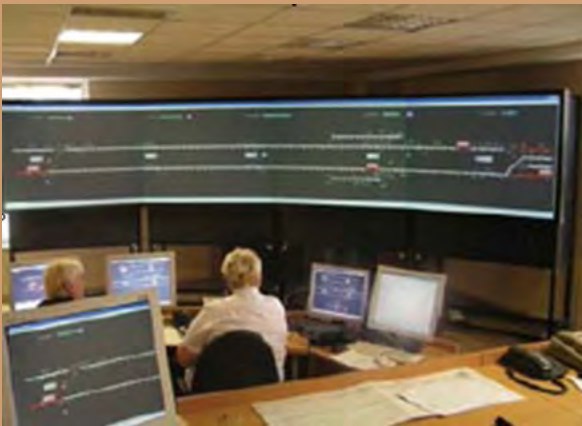
Dispatching Desk at Kazan Metro Operations
