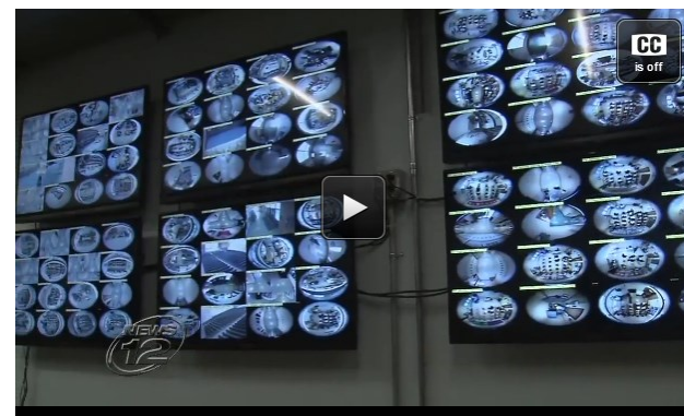
800 cameras implemented to cover school premise
